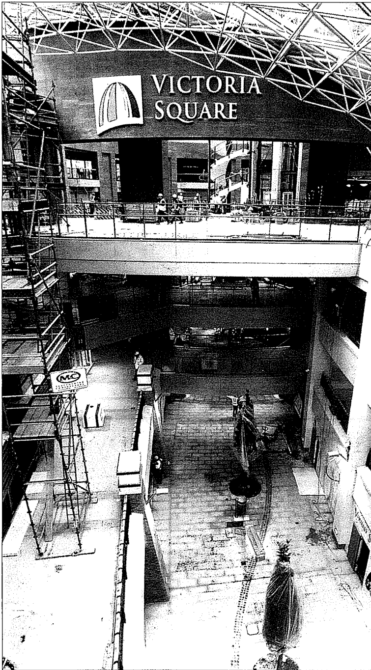
WORK IN PROGRESS: the Victoria Square development, viewed from Ann Street, will be opened next Thursday
