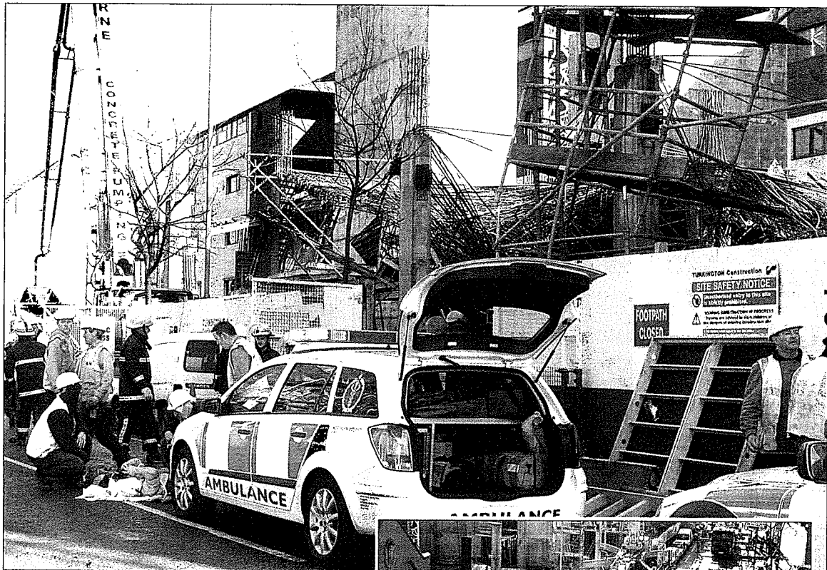
TREATMENT: rescue workers tend to an injured man
